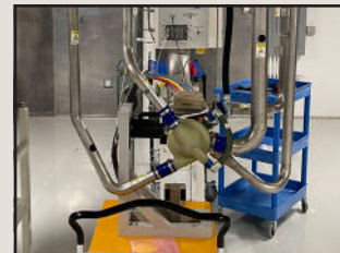
Motor Driven Compressor
